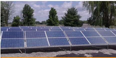
The ground mount solar array installed by SP&L for the Village of St. Paris, Ohio.
